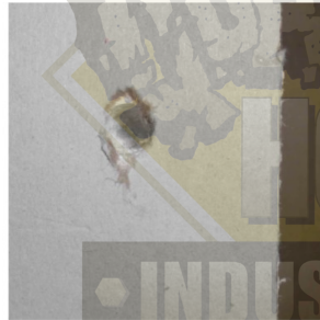
Look in hole to see if a stud has been hit
